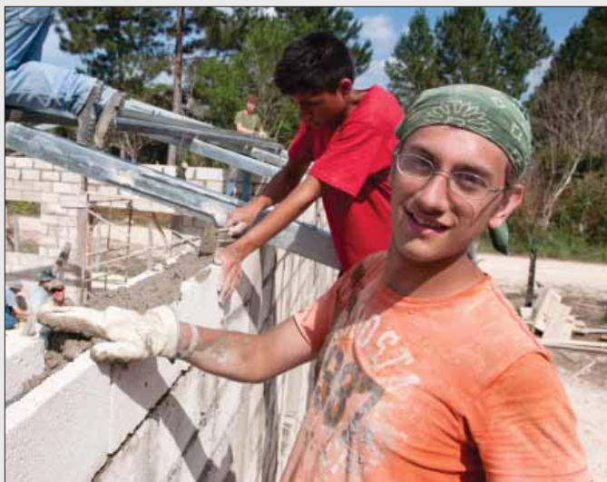
Home-school student Sklyer Bushnell adds concrete inside the top layer of blocks for a new church in Guatemala.
