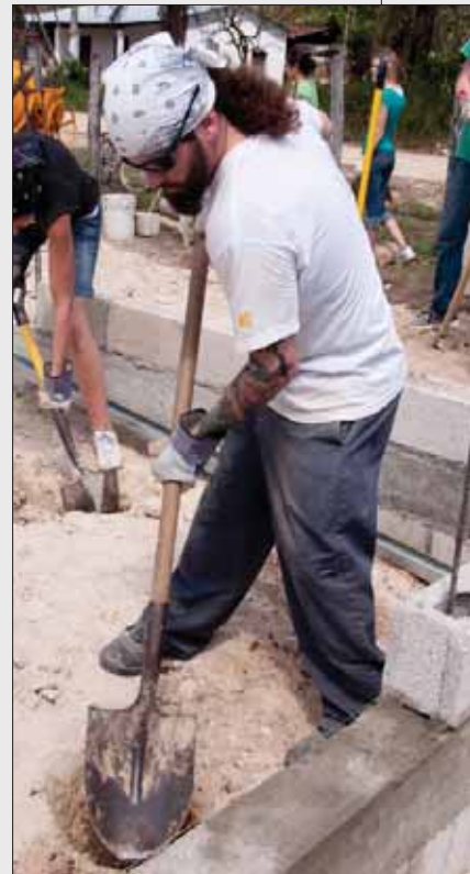
Former tattoo artist and alcoholic Justin Lathrop shovels dirt in preparation for a new church built in Poptun, Guatemala.
