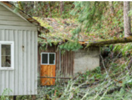
Falling trees during a winter storm that blew through in December damaged the roof of Camp Umpqua's lodge.
