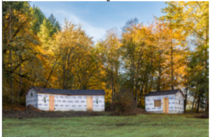
A new single cabin and a duplex in the boys' village still need some finishing touches to be ready for use.
