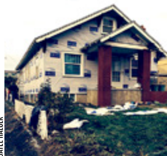
The little house is wrapped and ready for wood siding donated by Hy Mark Wood Products.
