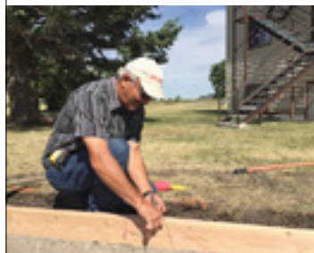
Marvin Herbel, class of 1965, checks a form for levelness before new sidewalks are poured.
