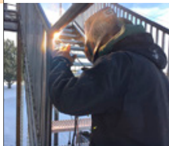
Randy Binder works on MEA fire escapes despite frigid temperatures. The fabrication project is scheduled to be complete by Alumni Weekend, April 14–16.
