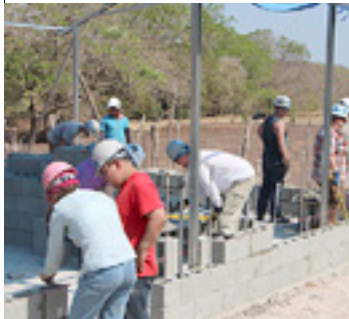
The AGA group hard at work adding walls to the One-Day Church.
